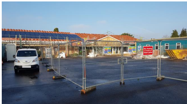
Top – Mile Cross Methodist Church in December 2021 with sign inset Above – Hellesdon Community Centre undergoing renovations in January 2022
